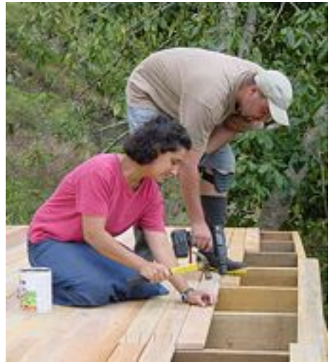
April Markley works on flooring for her house during a visit to Sakam village this summer.
